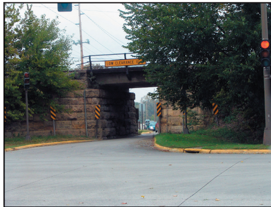
The underpass at Pammel St and Haber Rd currently allows only one direction of traffic through at a time. Project 4B (Elwood Drive Extension) would widen the underpass and reduce traffic on the ISU campus.
